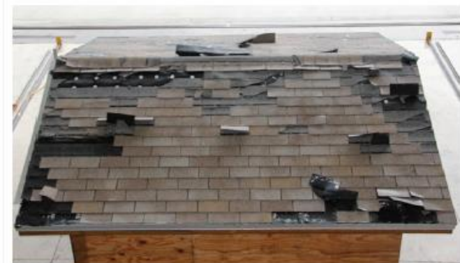
Treated deck after 145 mph, 180 degrees. Roof damage after the final test at the highest wind speed. The middle of the field suffered less damage compared to untreated deck.
