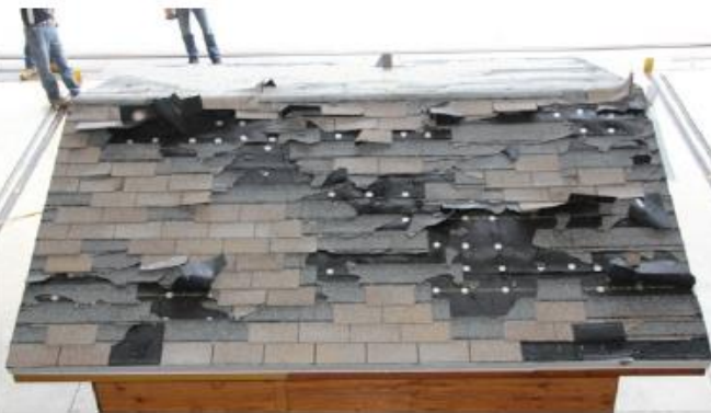
Untreated deck after 145 mph, 0 degrees. Roof damage after the final test at the highest wind speed.
