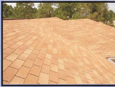
This is the same roof after it was sealed with Roof-Guard and the 2004 hurricanes
