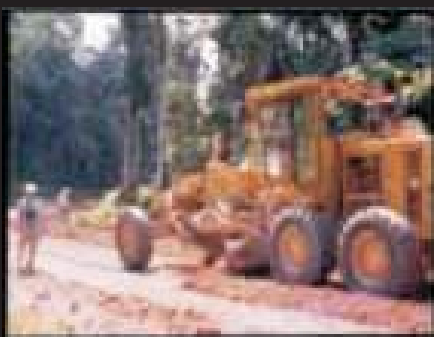
Installed in hi-plastic red clay reduced to near "0" and proctor of 98 in 24 hours. Traffic on this road as we worked
