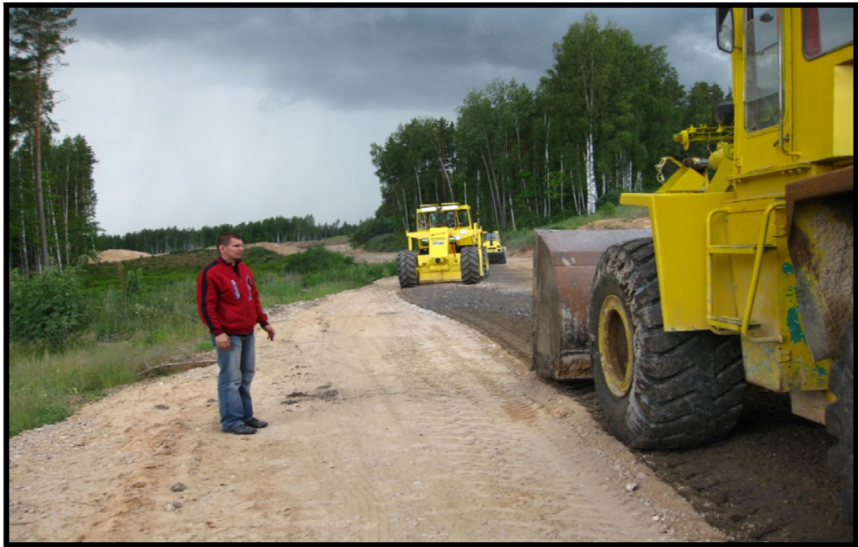
Figure 1 Installing M10+50/2001 with Bomag 122-2 at 15cm with application rate of 20 to 50m 3 /p/minute. This machine adjusts the proper optimum moisture and stabilizer content for perfect blended applications. The 15 ton vibratory roller comes right behind the application providing the finished road. The material used for this road was 25% clay, 75% crusher run of 15mm – or ½”- . It rained all night after the installation and in the morning the road maintained its integrity and density. No other product can claim this; “Guaranteed” .
